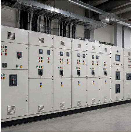
TURNKEY ELECTRICAL PROJECTS
