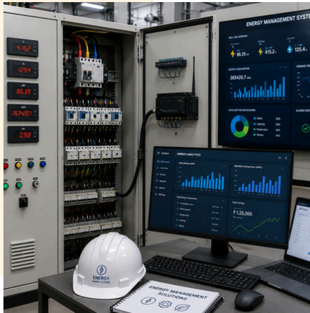
POWER DISTRIBUTION SYSTEMS
